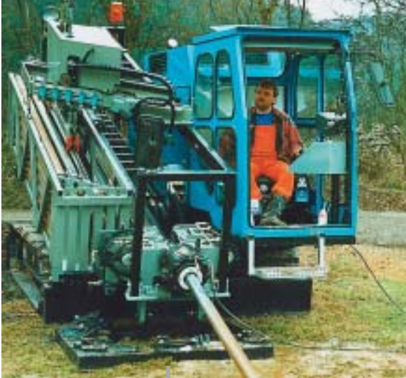
Pipes up to DN 600 are installed over a length of 500 m with the directional drilling system GRUNDODRILL.
